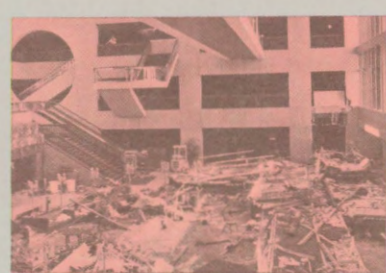
HOTEL DISASTER — Suspended walkways covered with people collapsed into the crowded lobby of the Hyatt Regency Hotel in Kansas City, killing 113 persons.
