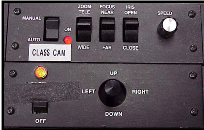
Classroom Camera Controls
